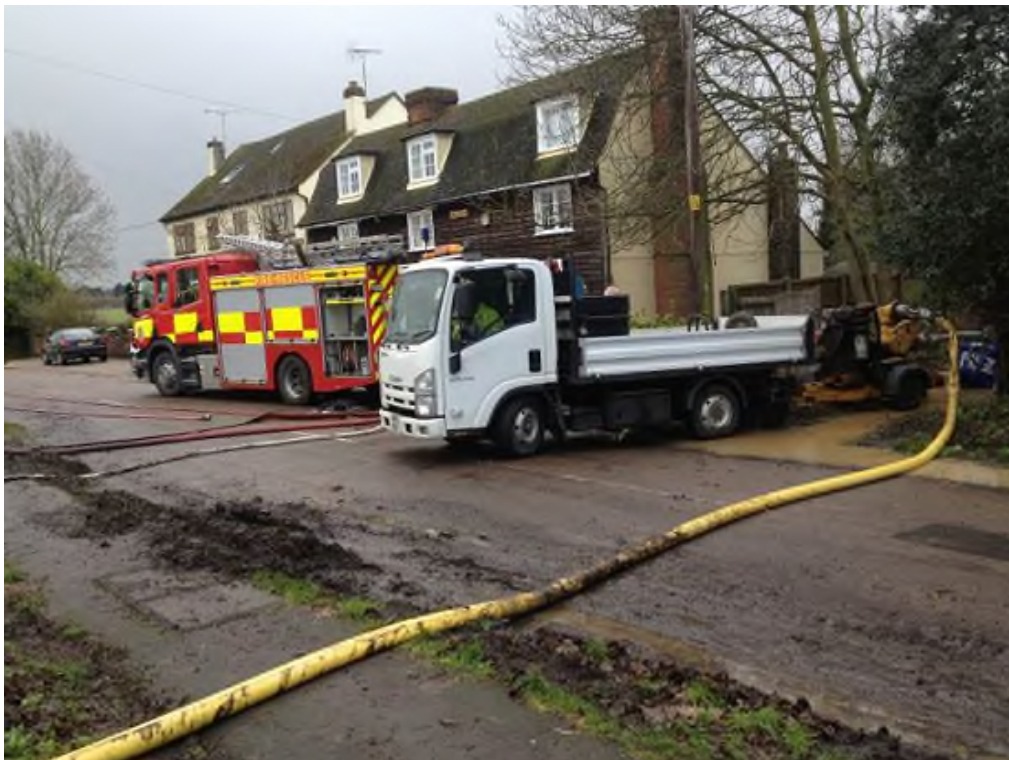
Figure 2: Emergency pumping of flood water
